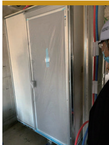
Figure 1.3.1.1-5 Modular bathroom with an RFID tag attached to its roof plate
