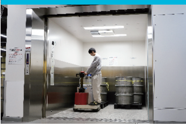
Figure 1.3.1.1-2 Lift in the facility
